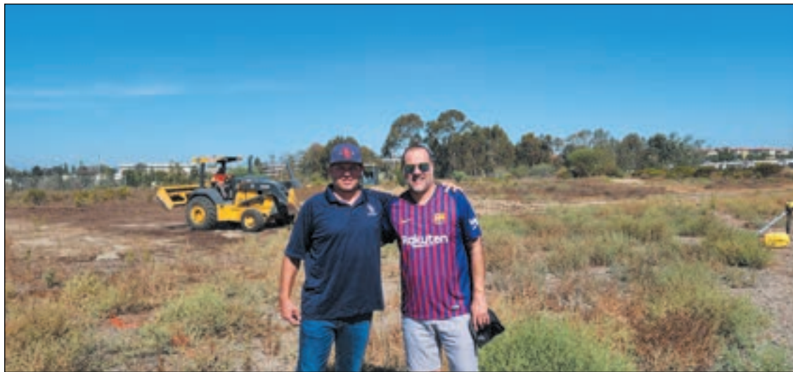
Lance Taschner (left) with Scripps Ranch High School Associate Principal Rudy Parra as construction of the new sand volleyball courts is underway on the school campus in the background. (courtesy of Lance Taschner)
