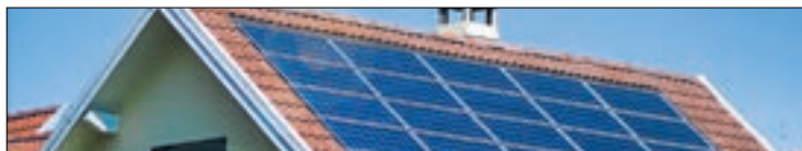
Numerous homes in Scripps Ranch now have rooftop solar panels.
