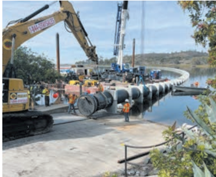
Construction of the Pure Water Program pipeline at Miramar Reservoir (courtesy of City of San Diego)
