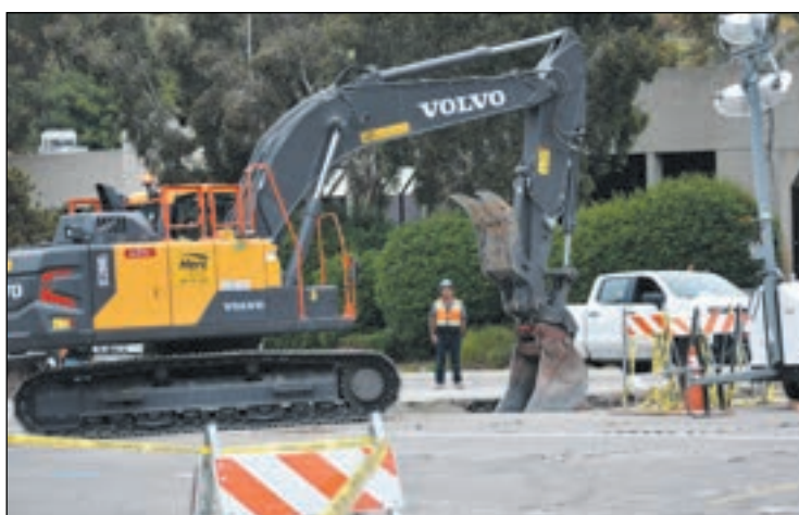
City workers repair a major water main break and sinkhole at the intersection of Scripps Lake Drive and Scripps Ranch Boulevard. (photo by John Gregory)
