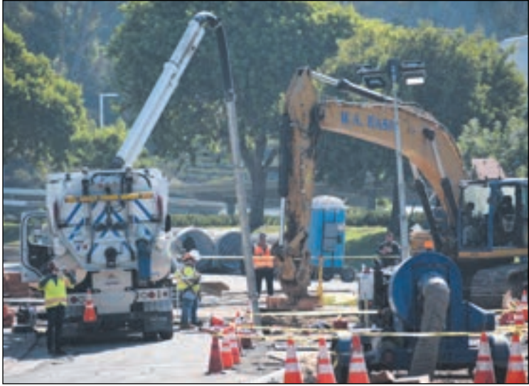
Construction and emergency personnel work around the site of a deadly trench accident on Aug. 28. (photo by John Gregory)
