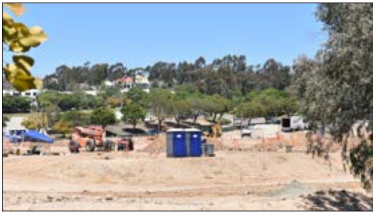
Preliminary work is underway at the site of the future Scripps Ranch Technology Park, situated between Scripps Ranch Boulevard and Hoyt Park Drive. (photo by John Gregory)
