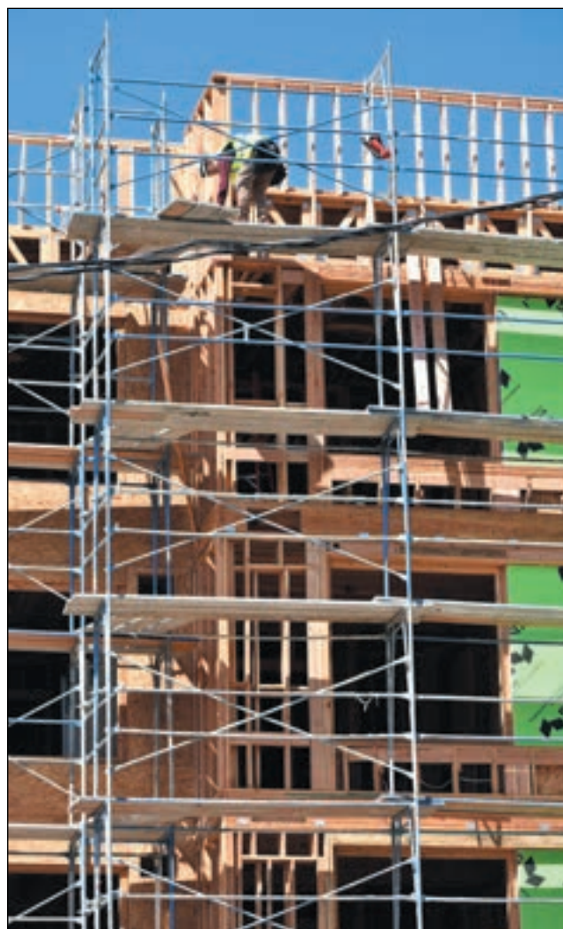
The Hub at Scripps Ranch, a mixed-use project at 9850 Carroll Canyon Road, is more than 50 percent complete and interior construction has begun. See page 5 (photo by John Gregory)
