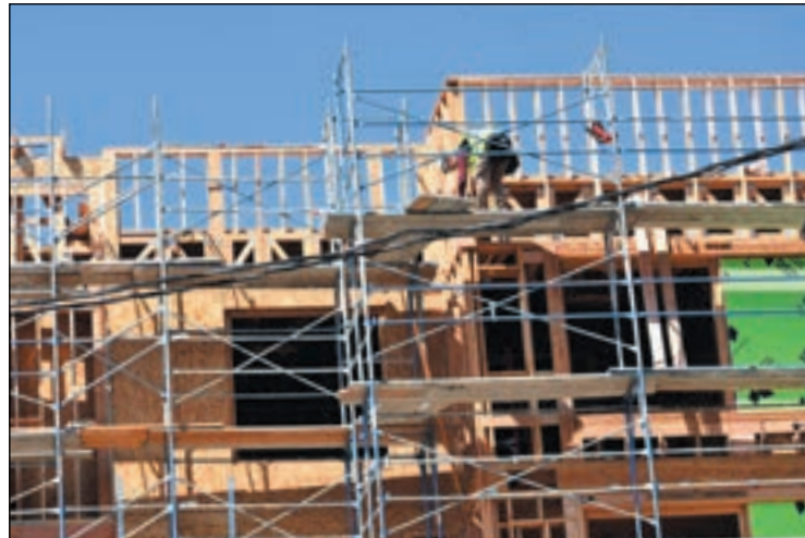
Framing is complete at Sudberry Properties' new redevelopment project, The Hub at Scripps Ranch, located on Carroll Canyon Road just east of I-15. The project will feature 260 luxury apartments, restaurants and retailers. (photo by John Gregory)
