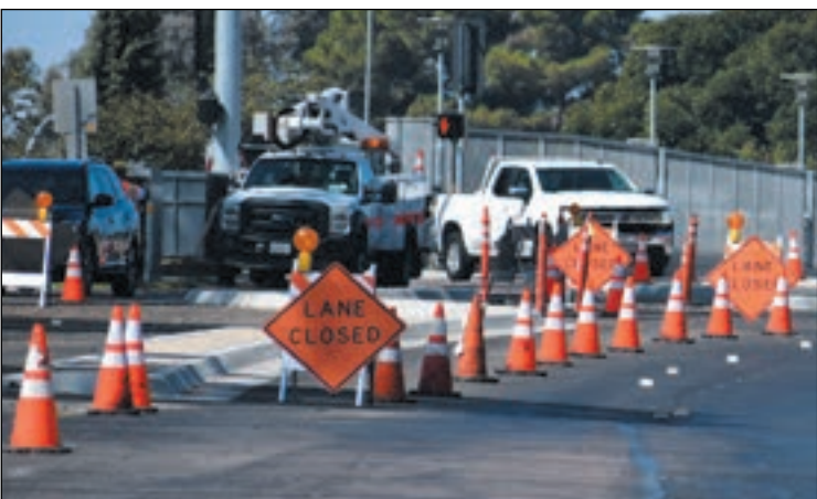
Potholing work to survey underground utilities, part of the massive Pure Water Program, continues along Carroll Canyon Road. See page 6 (photo by John Gregory)
