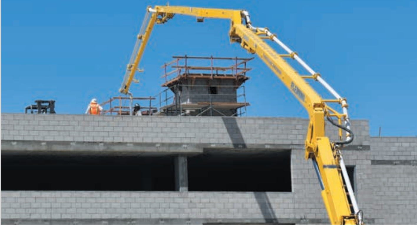
Construction of the controversial 264-unit mixed use joint occupancy apartment complex at 10380 Spring Canyon Road continues. This photo shows work at the rear of the complex. The Voice of Scripps Ranch organization was unsuccessful in halting the project after filing a lawsuit, but was awarded funds to drop the legal action, and continues to distribute the funds to community causes. See page 2 (photo by John Gregory)
