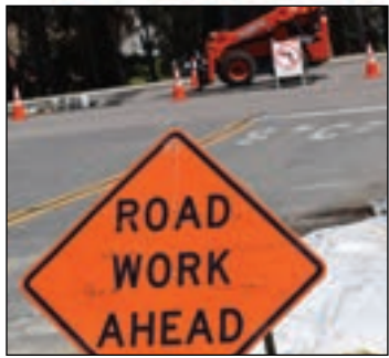
SDG&E works on a project along Scripps Ranch Boulevard next to Hoyt Park. (photo by John Gregory)
