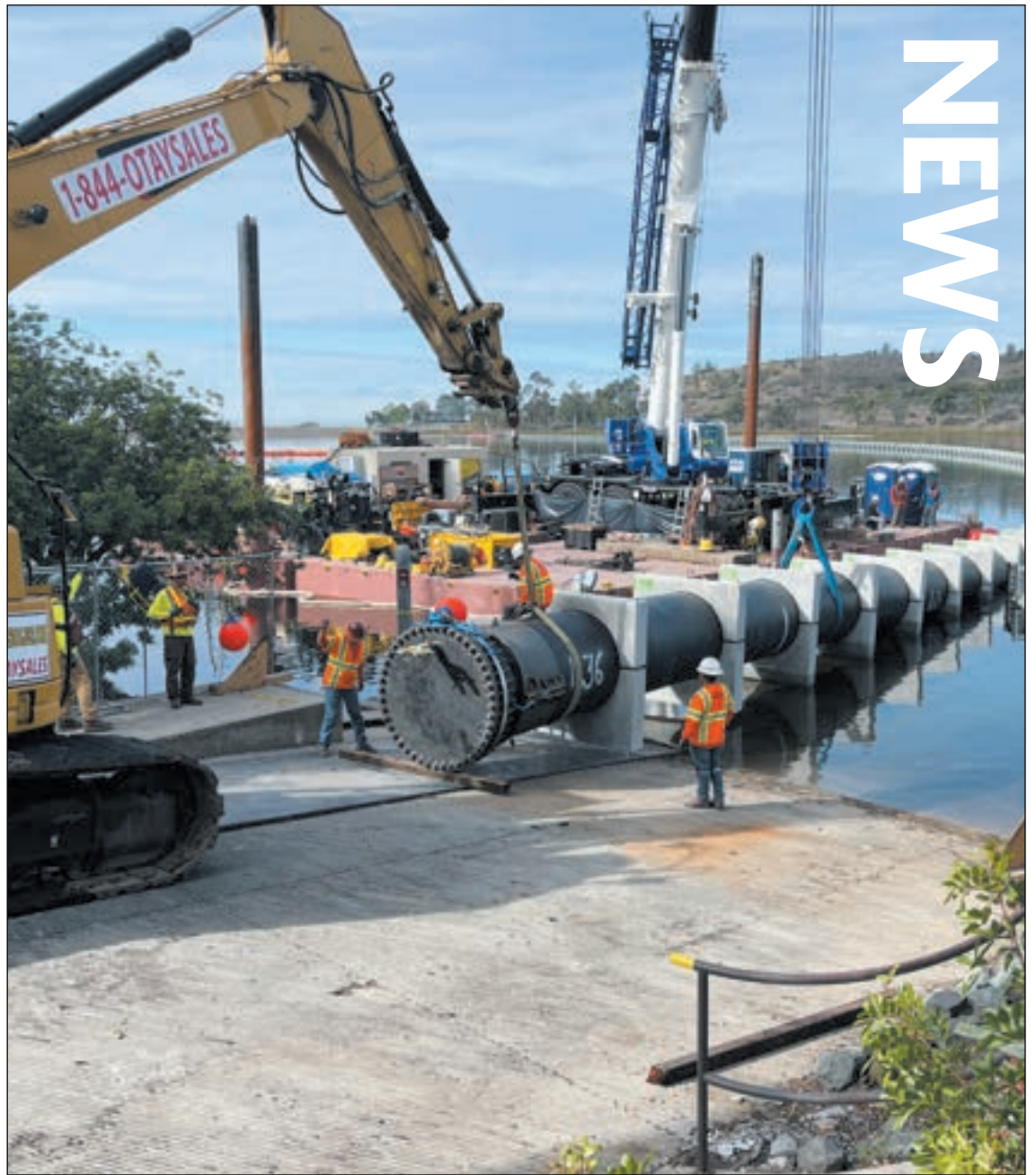
Construction of the Pure Water Program pipeline at Miramar Reservoir (courtesy of City of San Diego)
